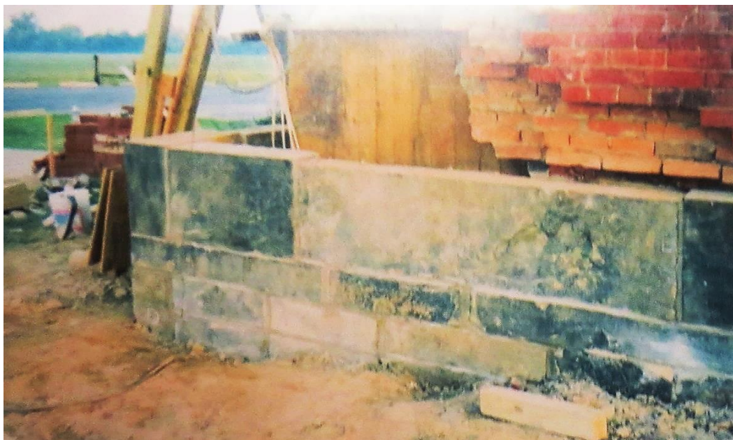
When repairing the corner of the building the original 8' long stone foundation slabs were clearly visible
